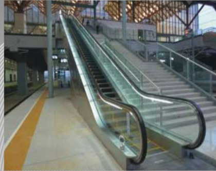
Suzhou Railway Station, China 9 units Elevators & 41 units Escalators
