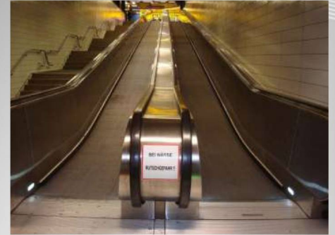
SWB Bonn. Metro, Germany 27 units Escalators & Travelators
