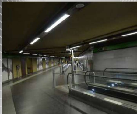
Milan Metro, Italy 2 units Escalators & 4 units Travelators
