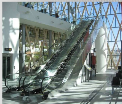
UMEA Railway Station, Sweden (10 units Escalators)
